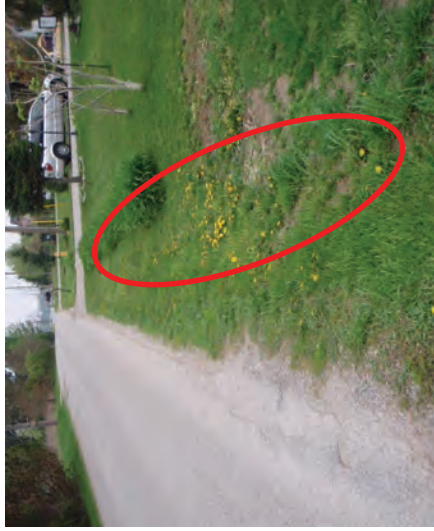
Shallow Roadside Ditch
