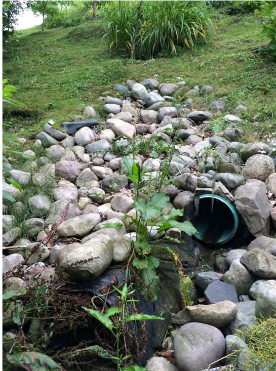
Photo 17, Culvert and outlet structures located at southeast corner of Springer Rd. and Longwoods Rd.
