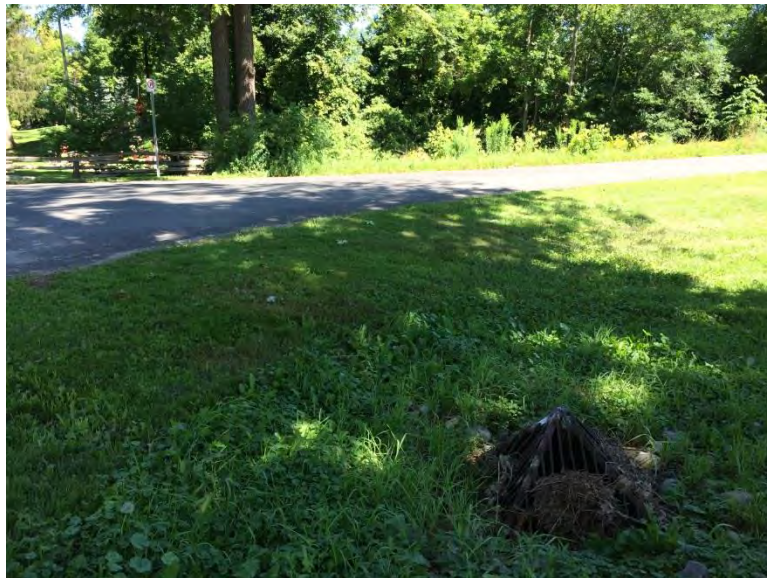
Photo 8, Raised inlet grate at intersection of Millcreek Lane and York Street.
