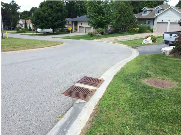
Photo 14, Inlet grates along Garden Avenue.
