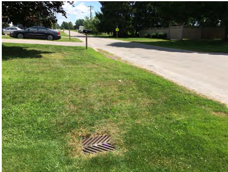
Photo 16, Inlet grate located along north side of Wellington Street, looking east along Wellington Street.
